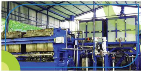
Waste Water Treatment Plan
