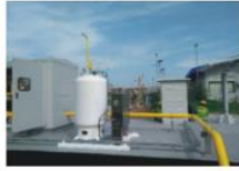
Odorizer Injection System
