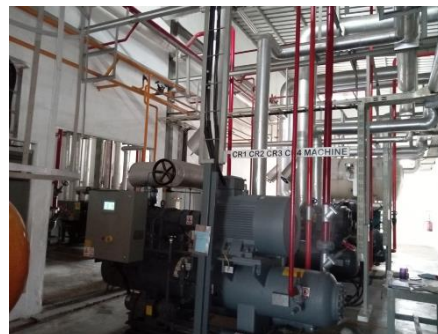
RUANGAN MESIN COLD ROOM
